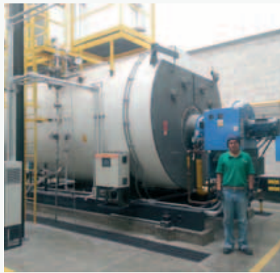
Ilama Felipe Ramos near the Myrigo Boiler located at Smurfit Kappa Atlacomulco Corrugated in Mexico.
